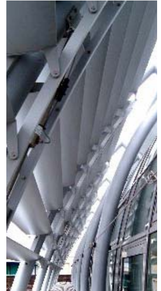
Example of mechanical louvers to control solar gain
